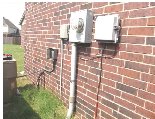
Figure 1: Service entrance ground
