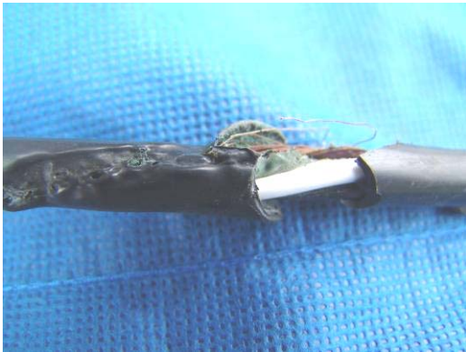
Figure 4: Ground conductor melted insulation
