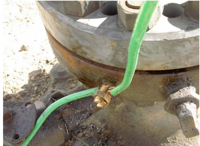
Fig. 3. Service post wellhead ground connection.
