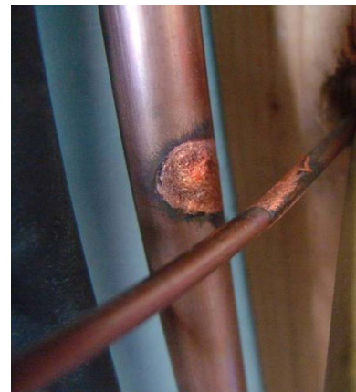
Fig. 6. Horizontal ground wire discharge to a vertical copper pipe.
